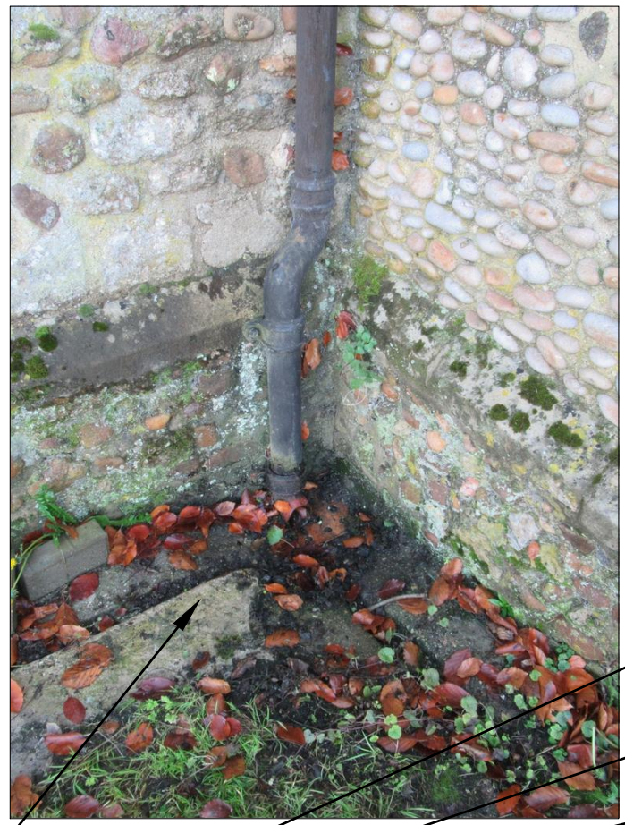
EXTG RWP No.8
