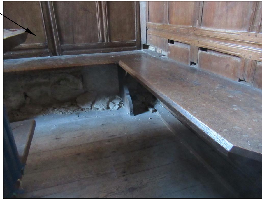
CHOIR STALLS - DETAIL SHOWING COLLAPSE AND SPOILED STONework
